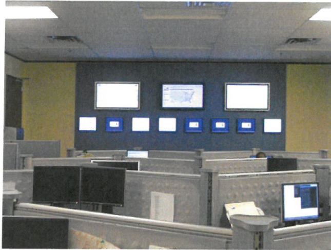
Network Operations Center (NOC)
